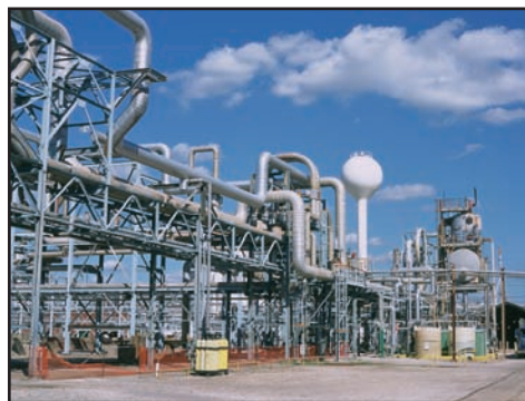
Shell Deer Park is home to a fully integrated refinery and petrochemical plant.
